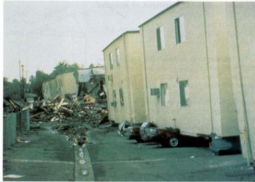
Northridge earthquake soft first story (parking level) damage. (Photo from: Brown, R.D., Jr., Lessons reaffirmed, extended, or revealed, Earthquakes and Volcanoes , Vol. 25, No. 2, 103-106, 1994)
