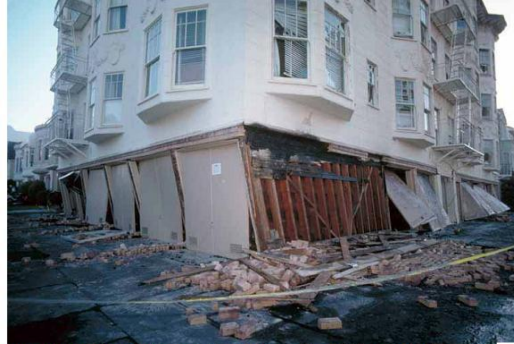
Loma Prieta earthquake damage in San Francisco. The soft first story is due to construction of garages in the first story and resultant reduction in shear strength. (Photo from: http://earthquake.usgs.gov/bytopic/photos.html )
